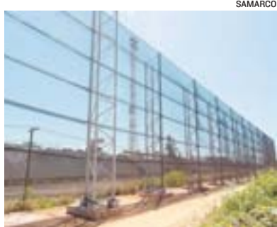
WIND FENCE: barreira de vento
